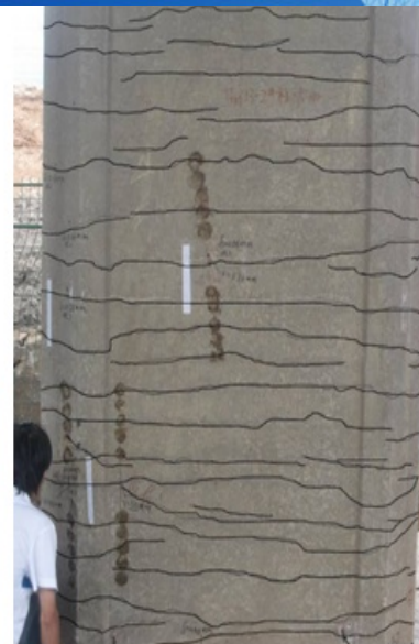
13#右墩外侧墩身裂缝
