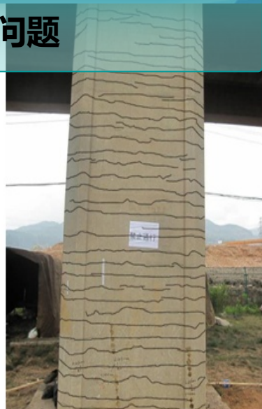
14#左墩外侧墩身裂缝
